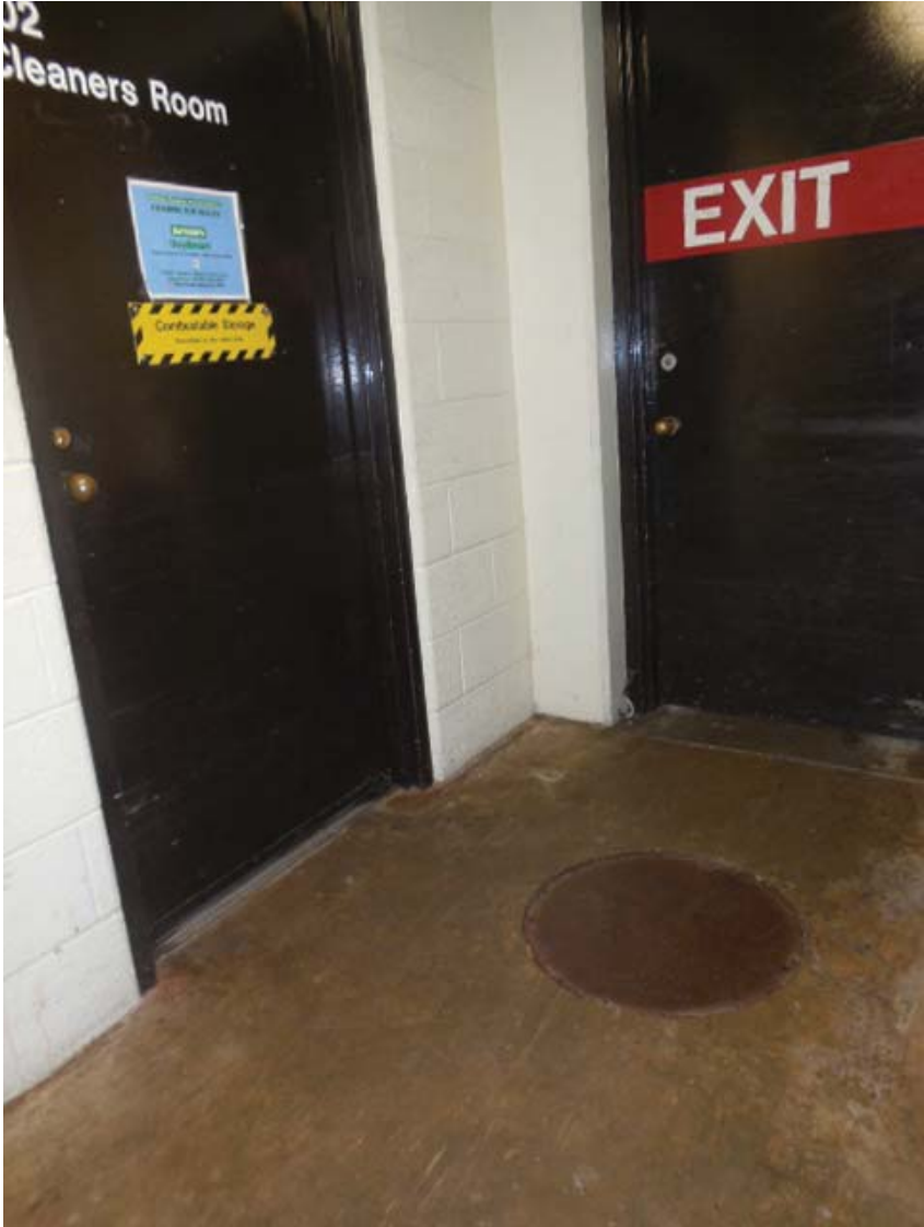
Photo #3: E07 West Hyattsville – Handhole in mezzanine level corridor
