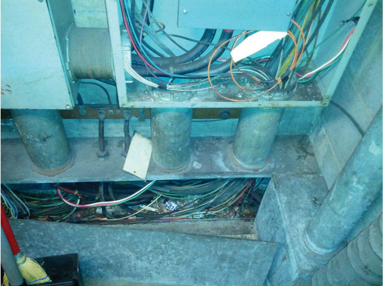
Archives Photo #4 – AFC Panel (MF) shared raceway (trough) with Panels MPO, M, ME, and MM (All in Room 203 Mezzanine Level)
