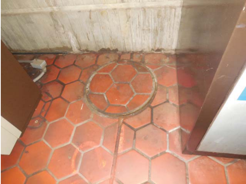
Photo #1: E08 Prince George's Plaza –Handhole in mezzanine floor
