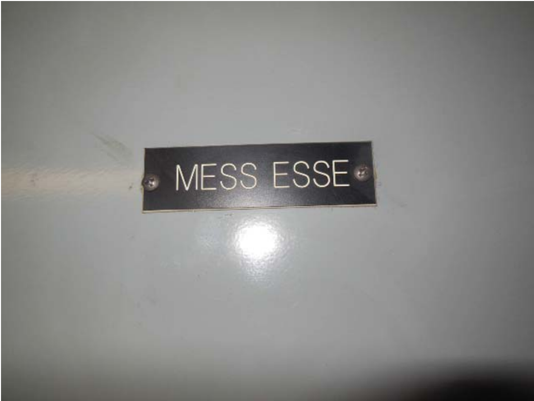
Picture 3: E05 Georgia Ave – AFC Panel MESS ESSE in room C213
