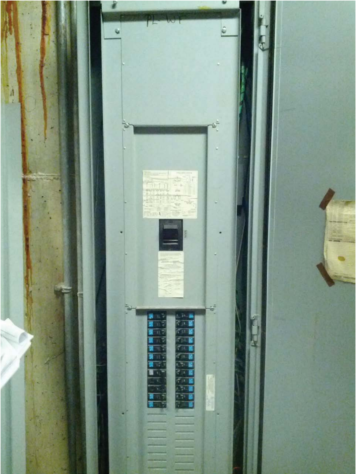
Picture 5: E03 U Street West - AFC Panel WF in Room 212
