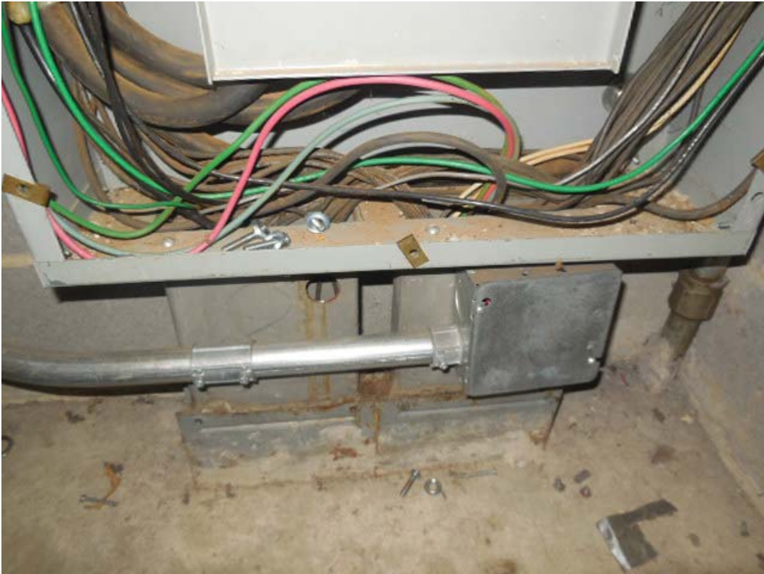
Photo #3: E09 College Park – Ducts at bottom of Panel F1 in Room C104
