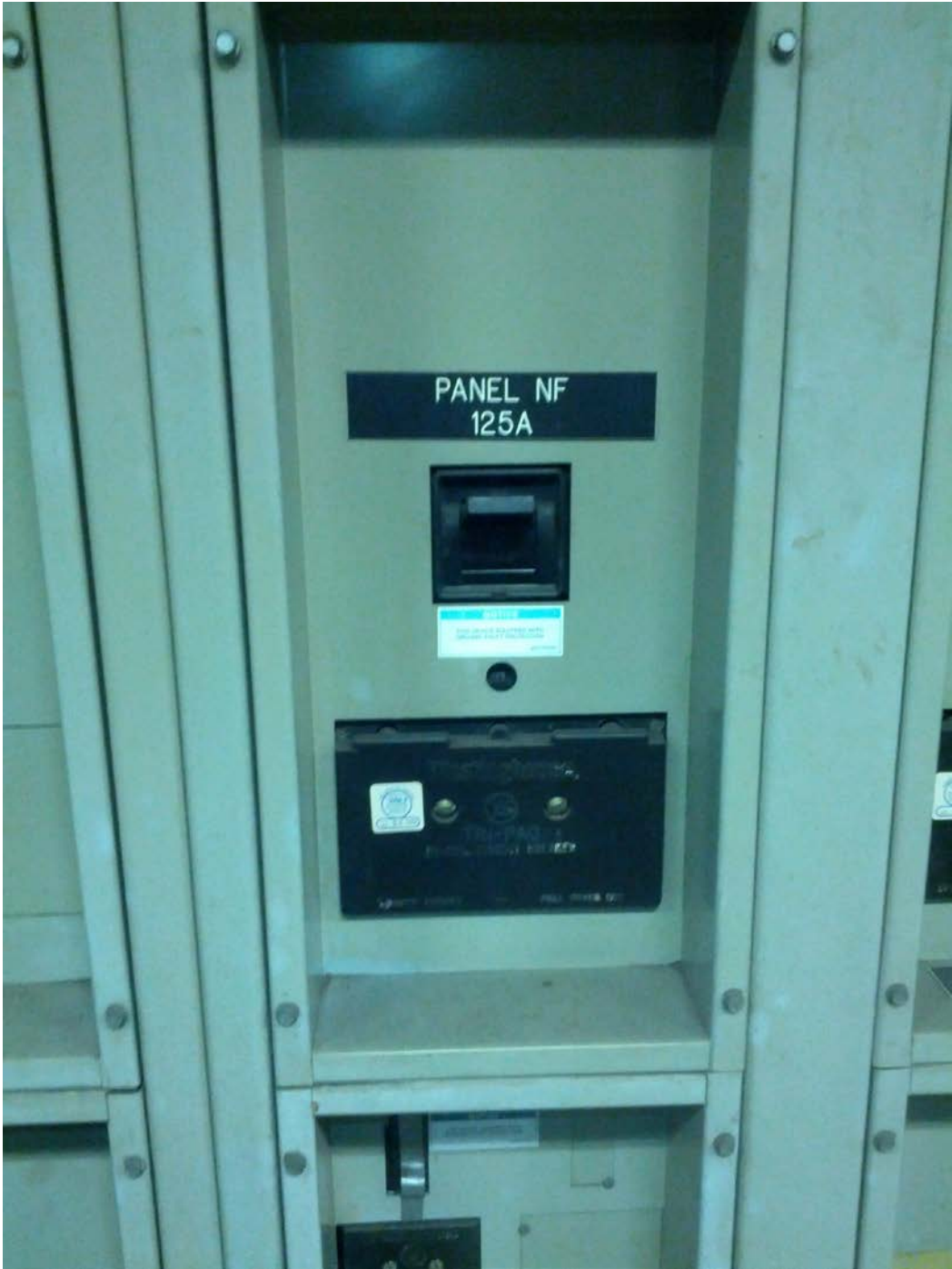
Photo #5: E02 Shaw-Howard U (North) – SWBD breaker for Panel NF in room 223
