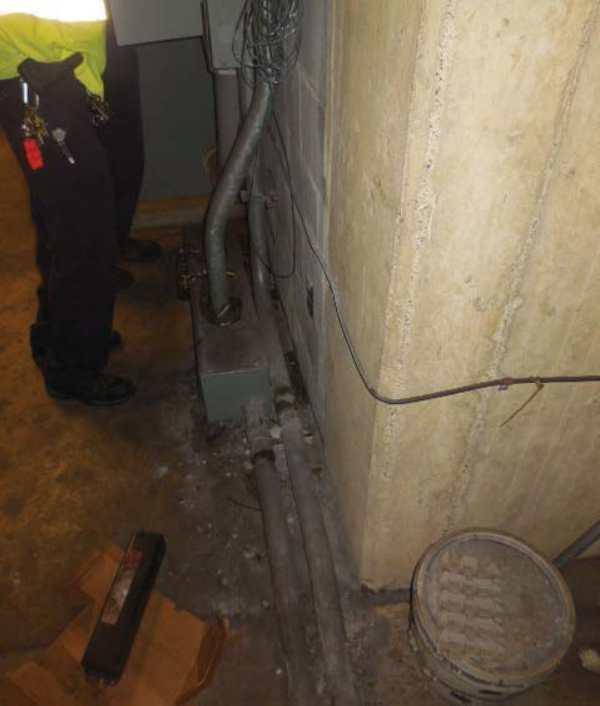
Pictures 5-7: E05 Georgia Ave – AFC Panel MESS ESSE in room C213, bottom conduits
