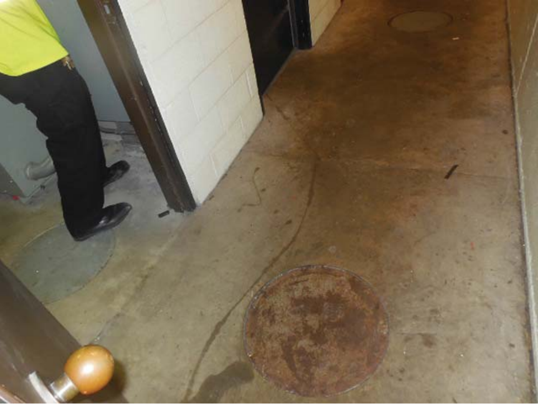
Photo #2: E09 College Park – Handholes in hallway
