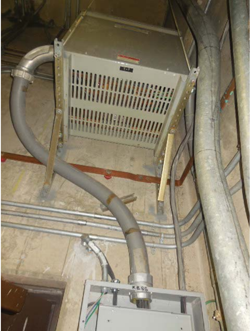
Photo #3: E08 Prince George's Plaza – Top of Panel KESS in room 210
