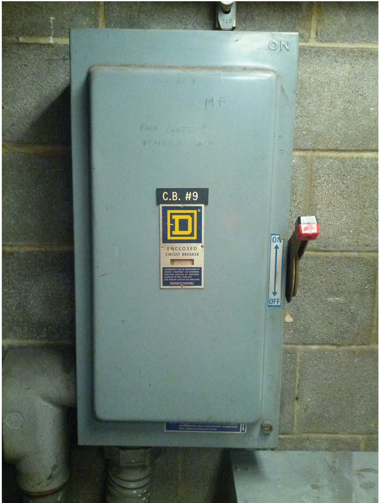
Archives Photo #2 – Disconnect Switch “Disc. MF” for AFC Panel (MF) - Room 203 (Mezzanine Level)
