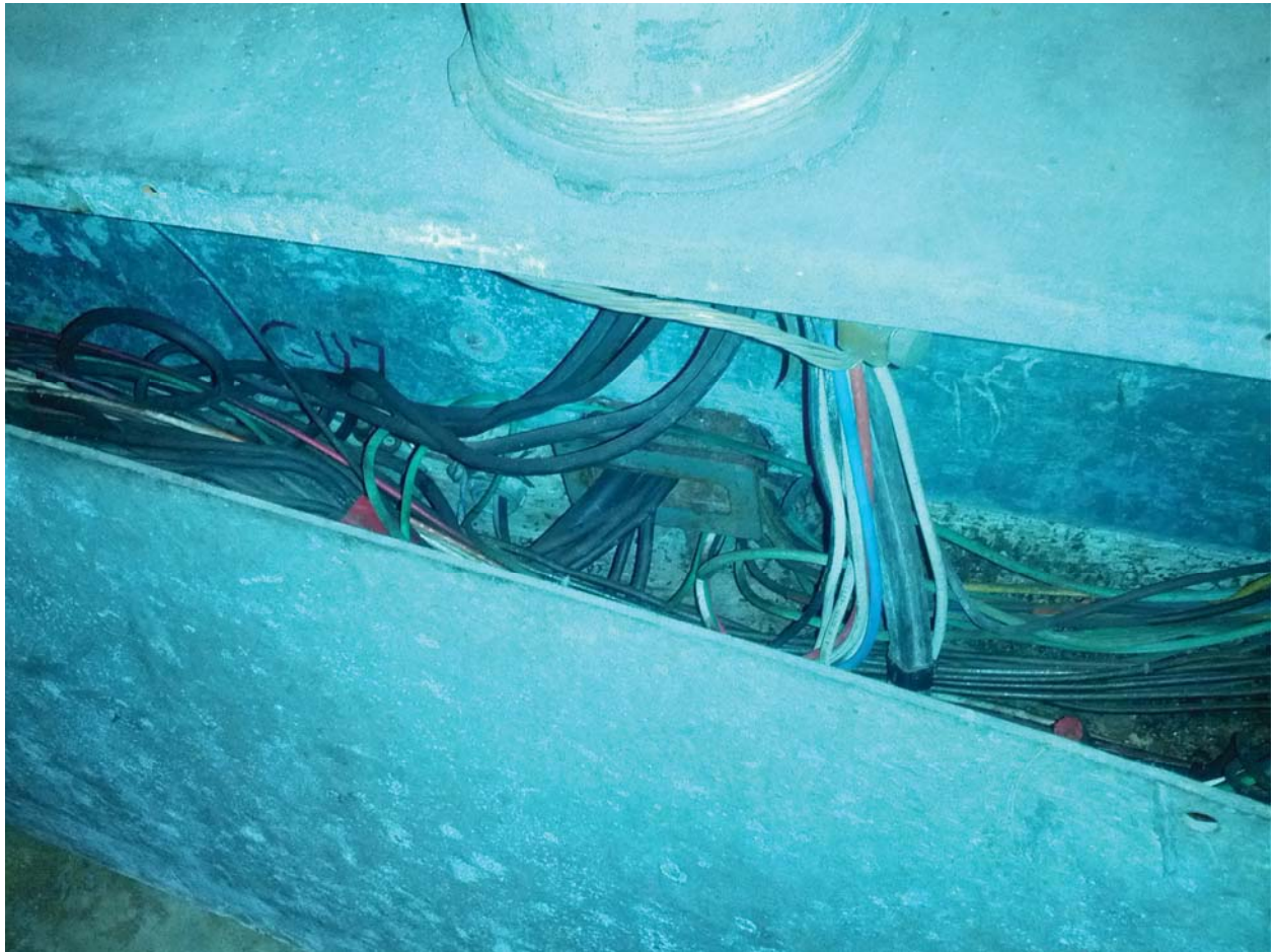
Archives Photo #5 – AFC Panel (MF) shared raceway (trough) with Panels MPO, M, ME, and MM (All in Room 203 Mezzanine Level)
