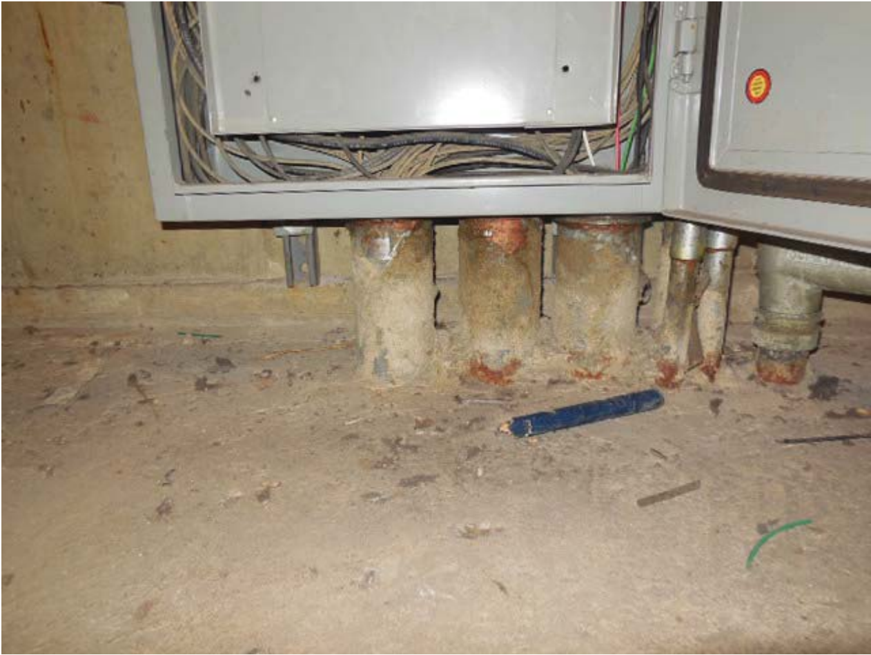
Picture 7: E03 U Street West - AFC Panel WF bottom conduits in Room 212
