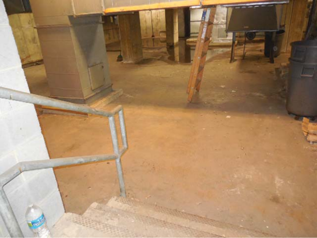
Picture 11: E03 U Street West – Standing water in room adjacent to AFC Panel
