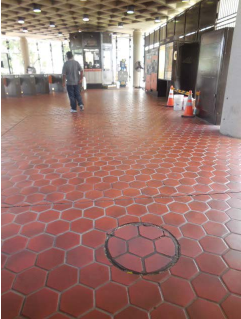
Photo #1: E07 West Hyattsville – Handhole in mezzanine floor
