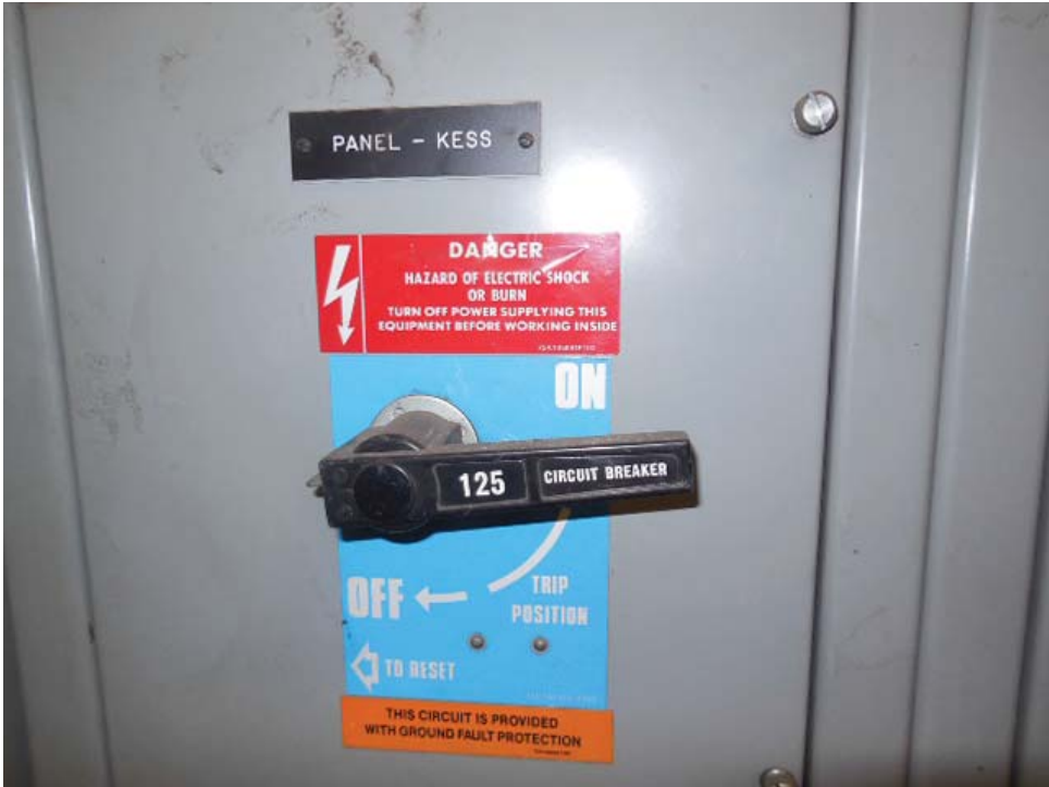
Photo #5: E08 Prince George's Plaza – SWBD breaker for Panel KESS in room 130 near track#1
