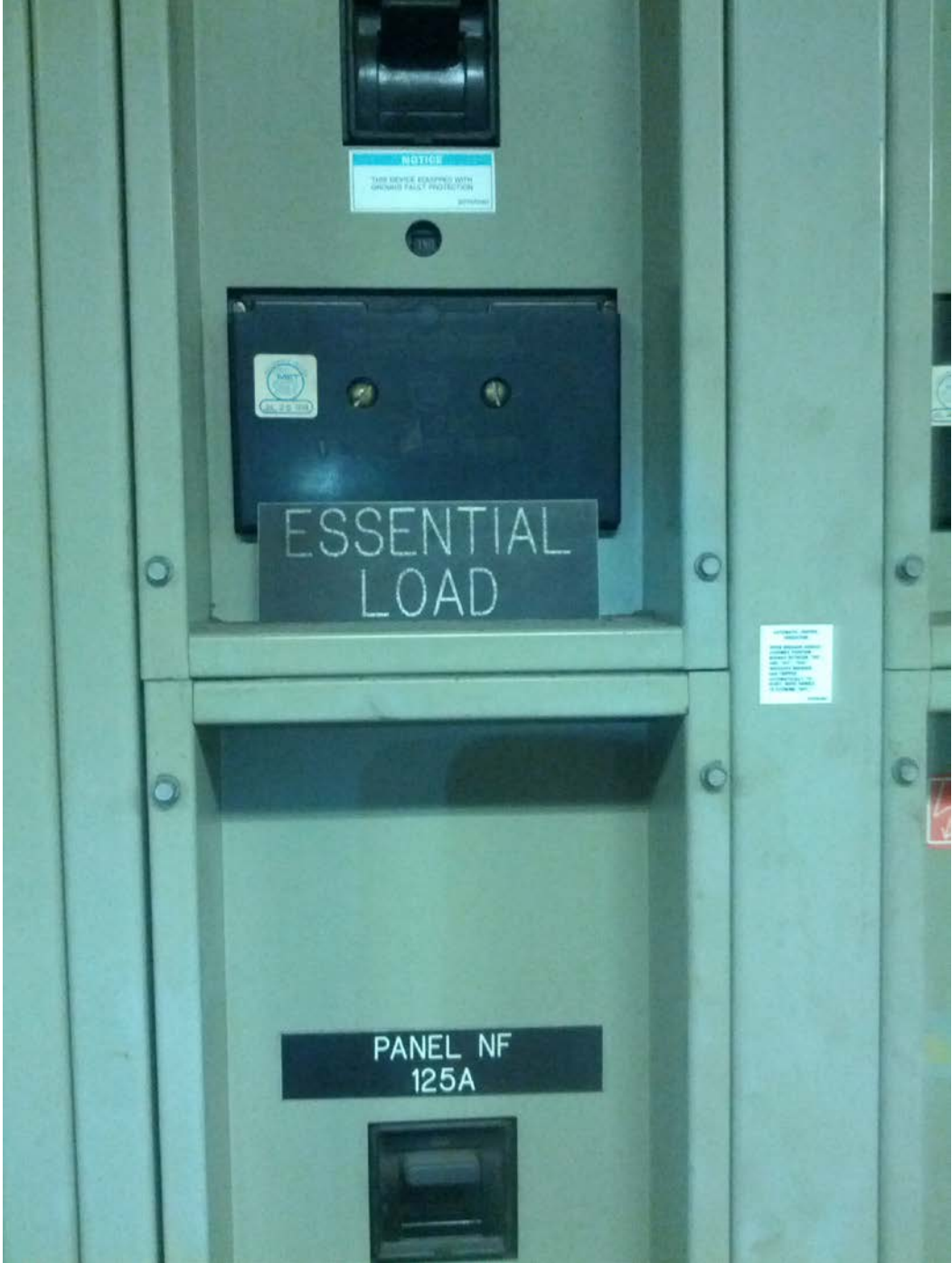
Photo #6: E02 Shaw-Howard U (North) – SWBD breaker for Panel NF in room 223
