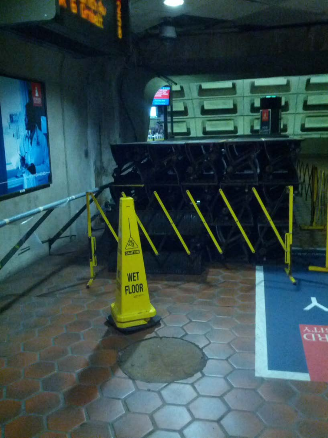
Photo #1: E02 Shaw-Howard U (North) – Handhole in mezzanine floor
