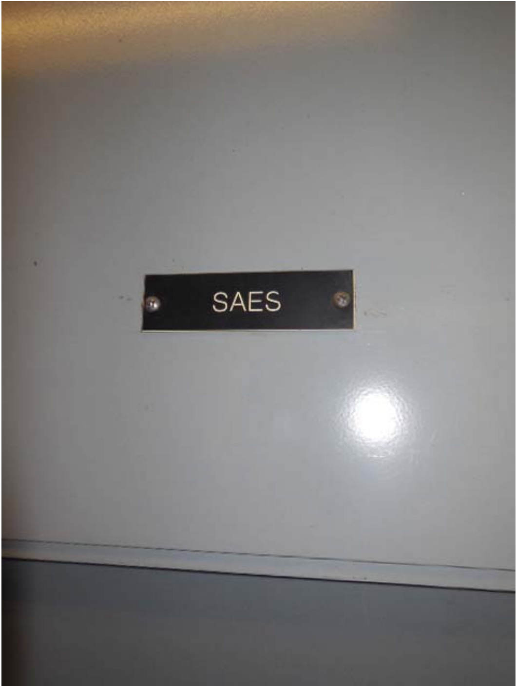
Picture 9: E05 Georgia Ave – Panel SAES in room C219
