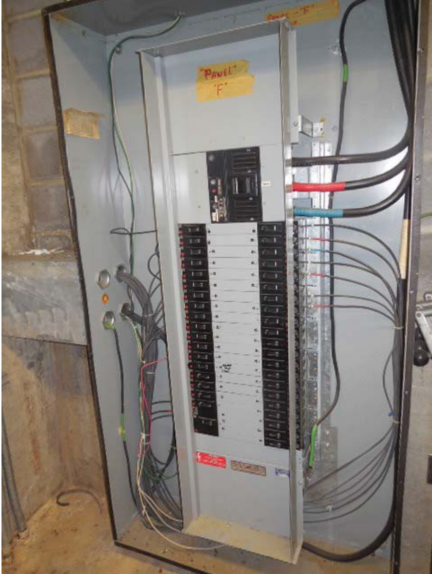
Photo #5: E07 West Hyattsville – Panel F in Room 108
