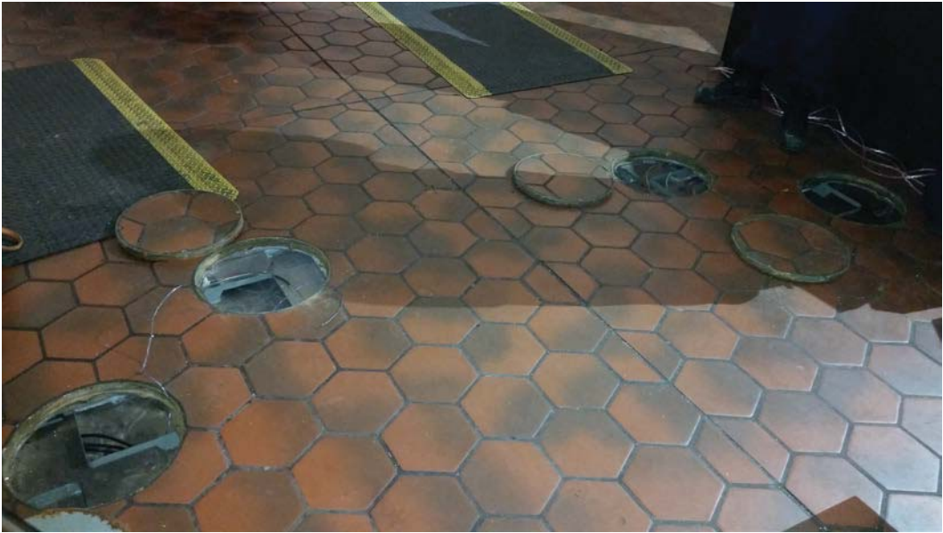
Picture 1: E05 Georgia Ave – Handholes on paid-side of mezzanine for faregate duct access
