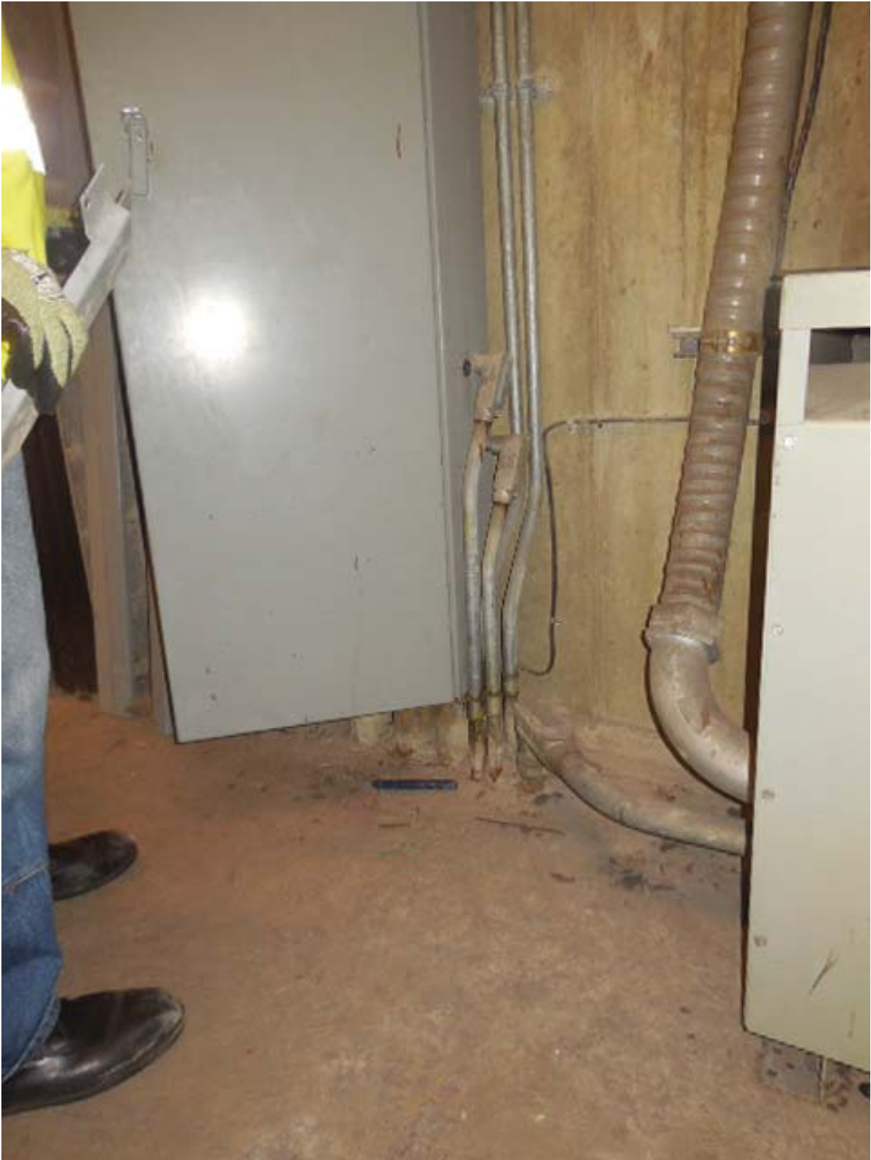
Picture 4: E03 U Street West - AFC Panel WF in Room 212
