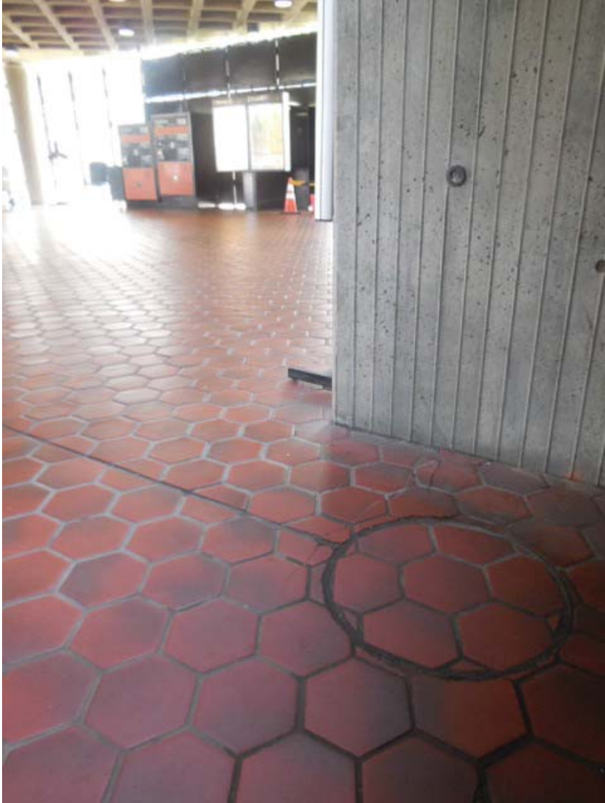
Photo #2: E07 West Hyattsville – Handhole in mezzanine floor
