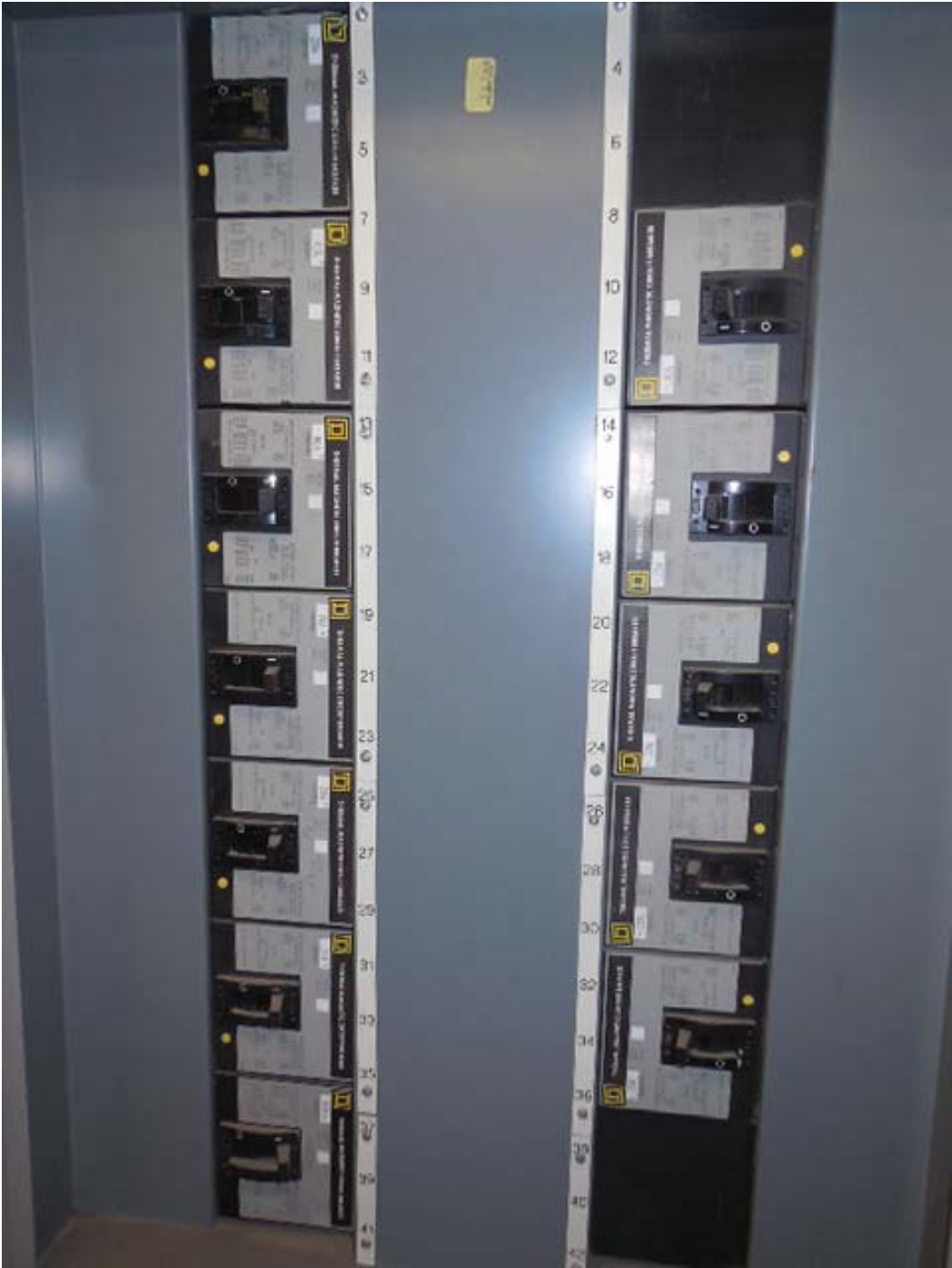
Picture 10: E05 Georgia Ave – Panel SAES in room C219, Circuits 37,39,41
