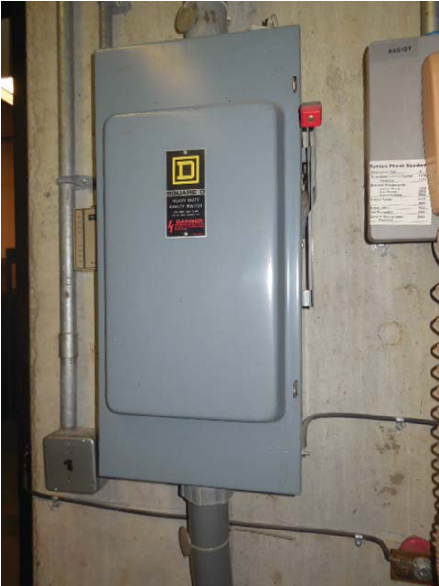
Photo #5: E10 Greenbelt – Disconnect Switch in Room C106
