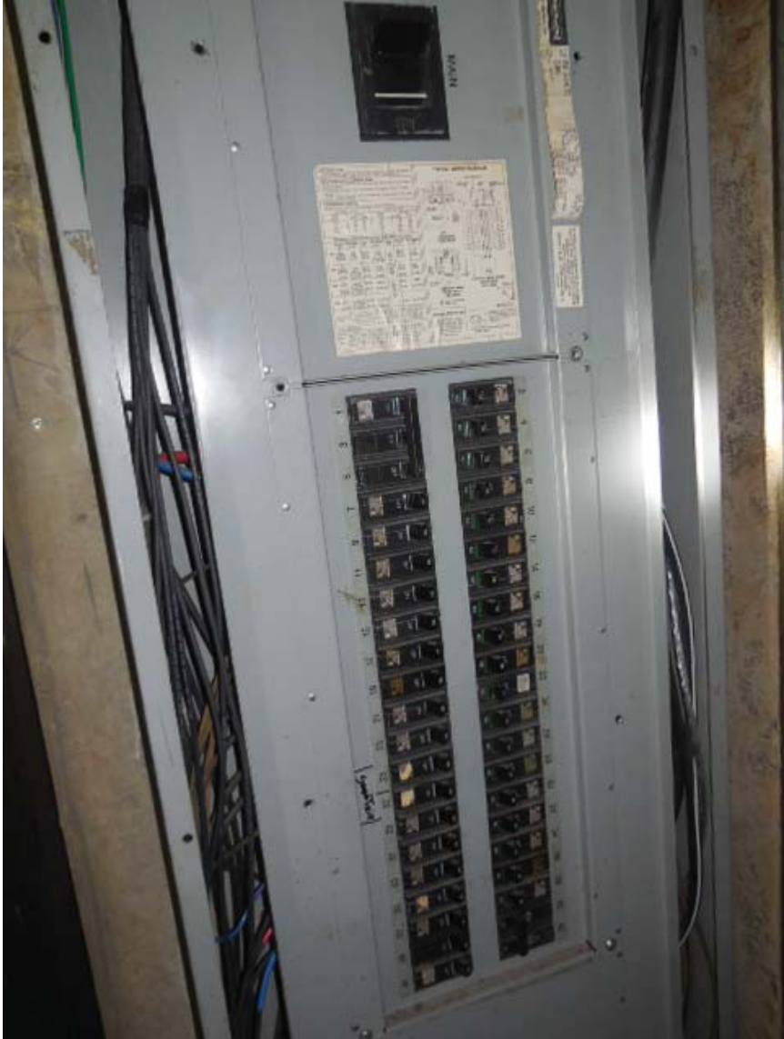
Photo #3: E08 Prince George's Plaza – Panel KESS in room 210
