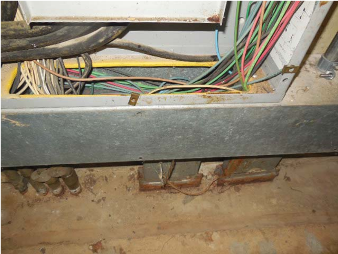
Photo #4: E10 Greenbelt – Ducts below Panel FF in Room C106
