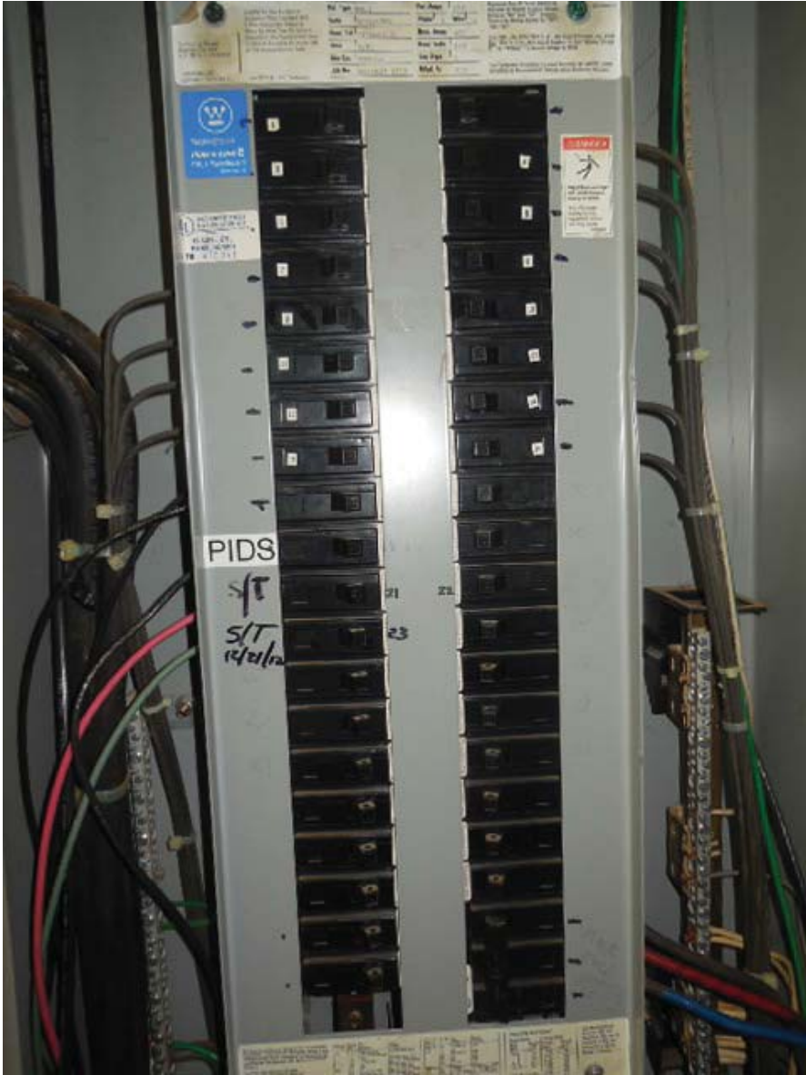
Photo #5: E09 College Park – Panel F1 in Room C104
