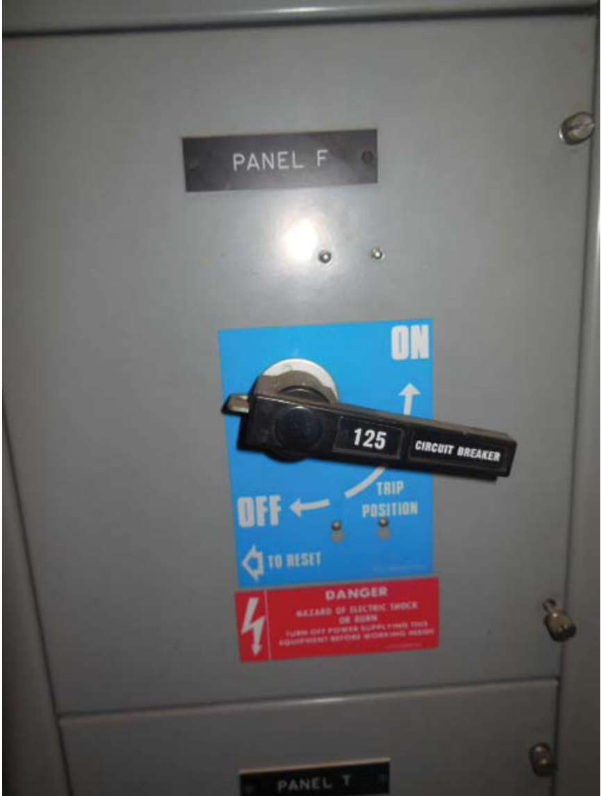
Photo #7: E07 West Hyattsville – SWBD A breaker for Panel F in Room 108
