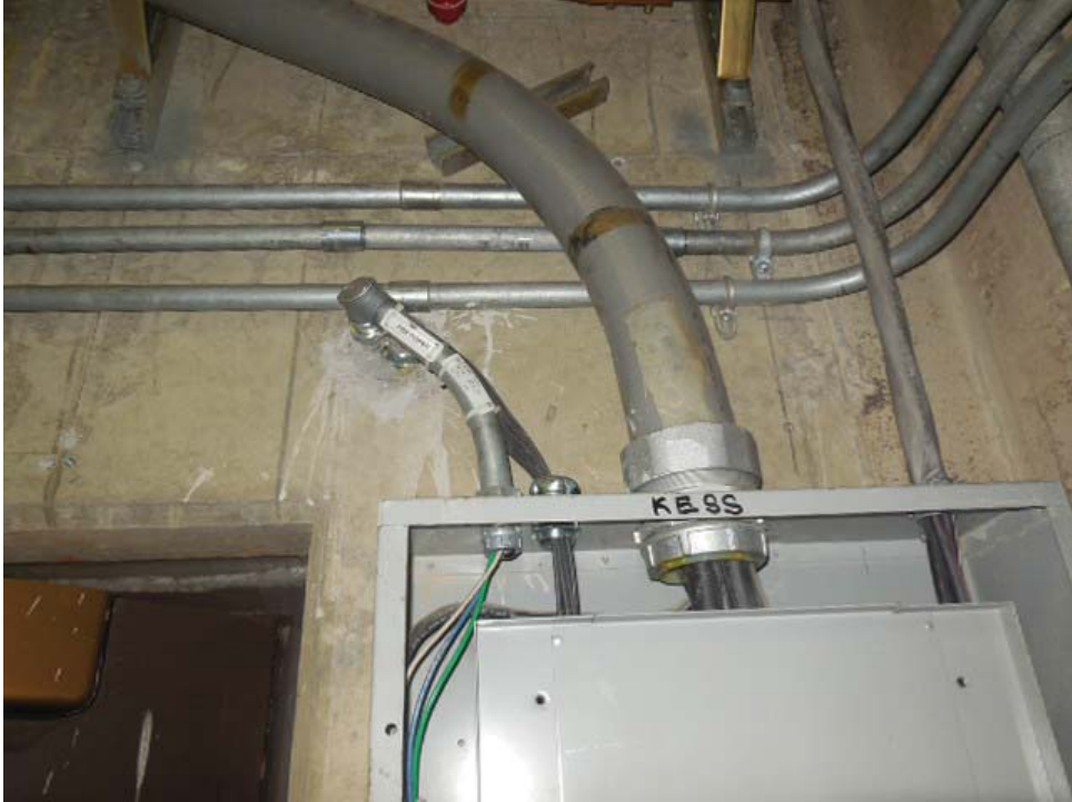
Photo #4: E08 Prince George's Plaza – Panel KESS in room 210
