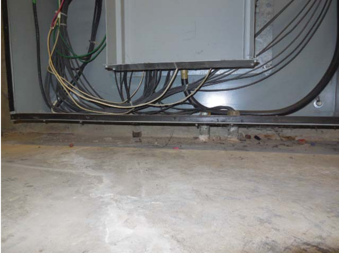
Photo #4: E07 West Hyattsville – Panel F in Room 108
