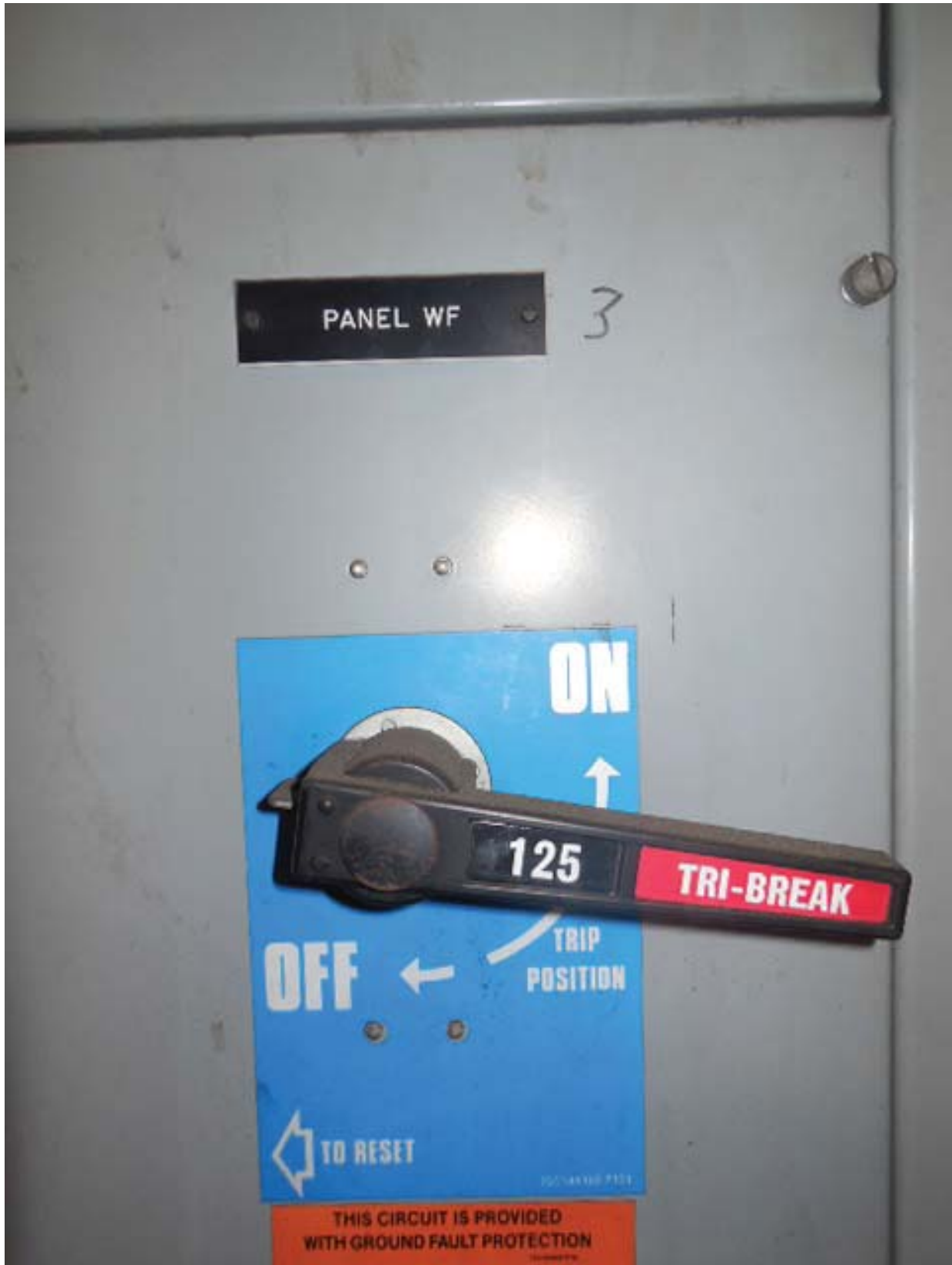
Picture 10: E03 U Street West – Essential SWBD – Panel WF Circuit 3
