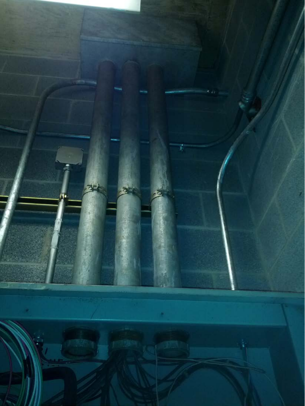
Photo #2: E02 Shaw-Howard U (North) – Pullbox and top of panel NF in room 205
