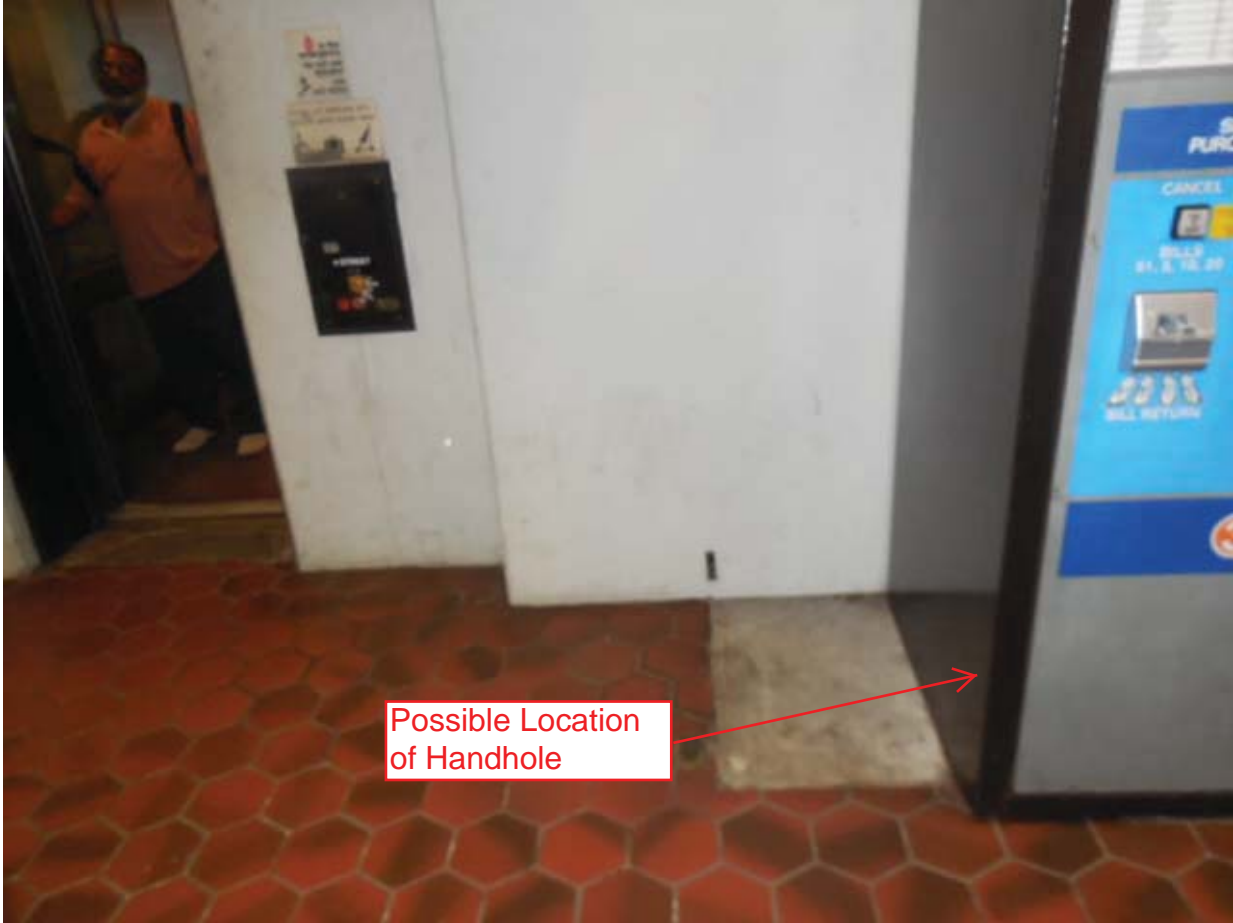
Archives Photo #7 – Location of Handhole noted on AFC As-Built Plan, but it could not be found.
