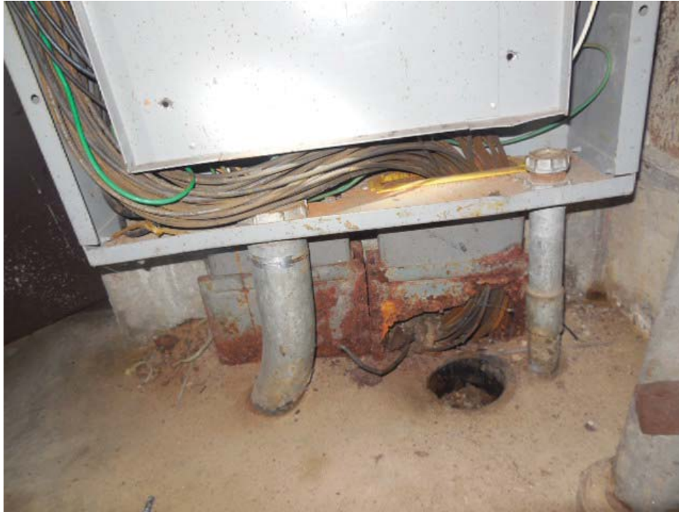
Photo #2: E08 Prince George's Plaza – Bottom of Panel KESS in room 210
