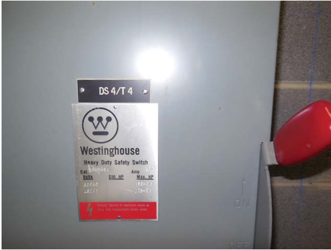
Photo #7: E09 College Park – Disconnect Switch DS4/T4 in Room C104
