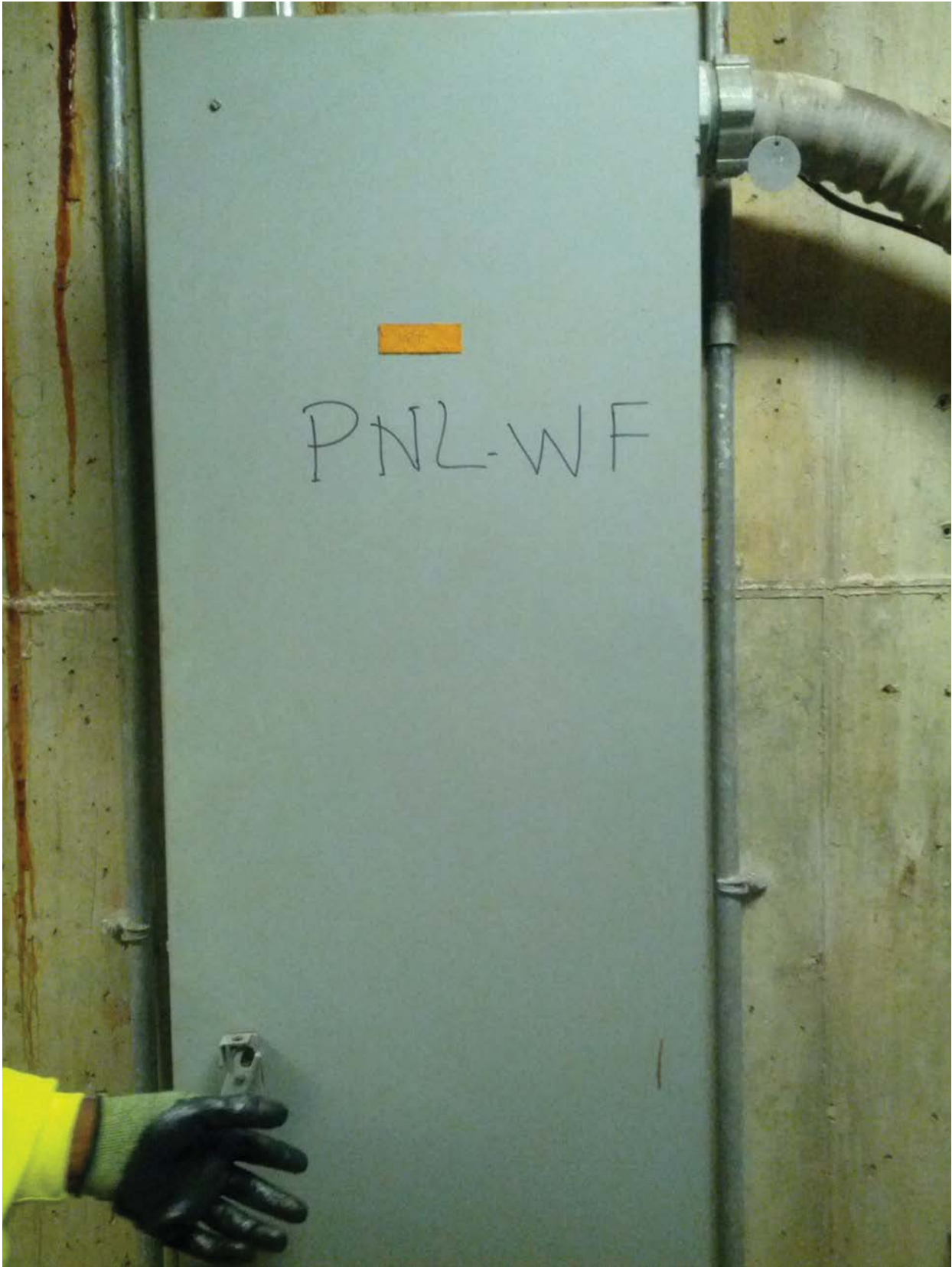
Picture 3: E03 U Street West - AFC Panel WF in Room 212
