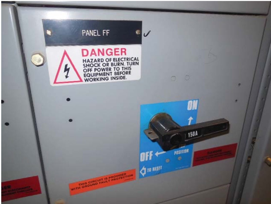
Photo #6: E10 Greenbelt – SWBD #2 breaker for Panel FF in Room C106
