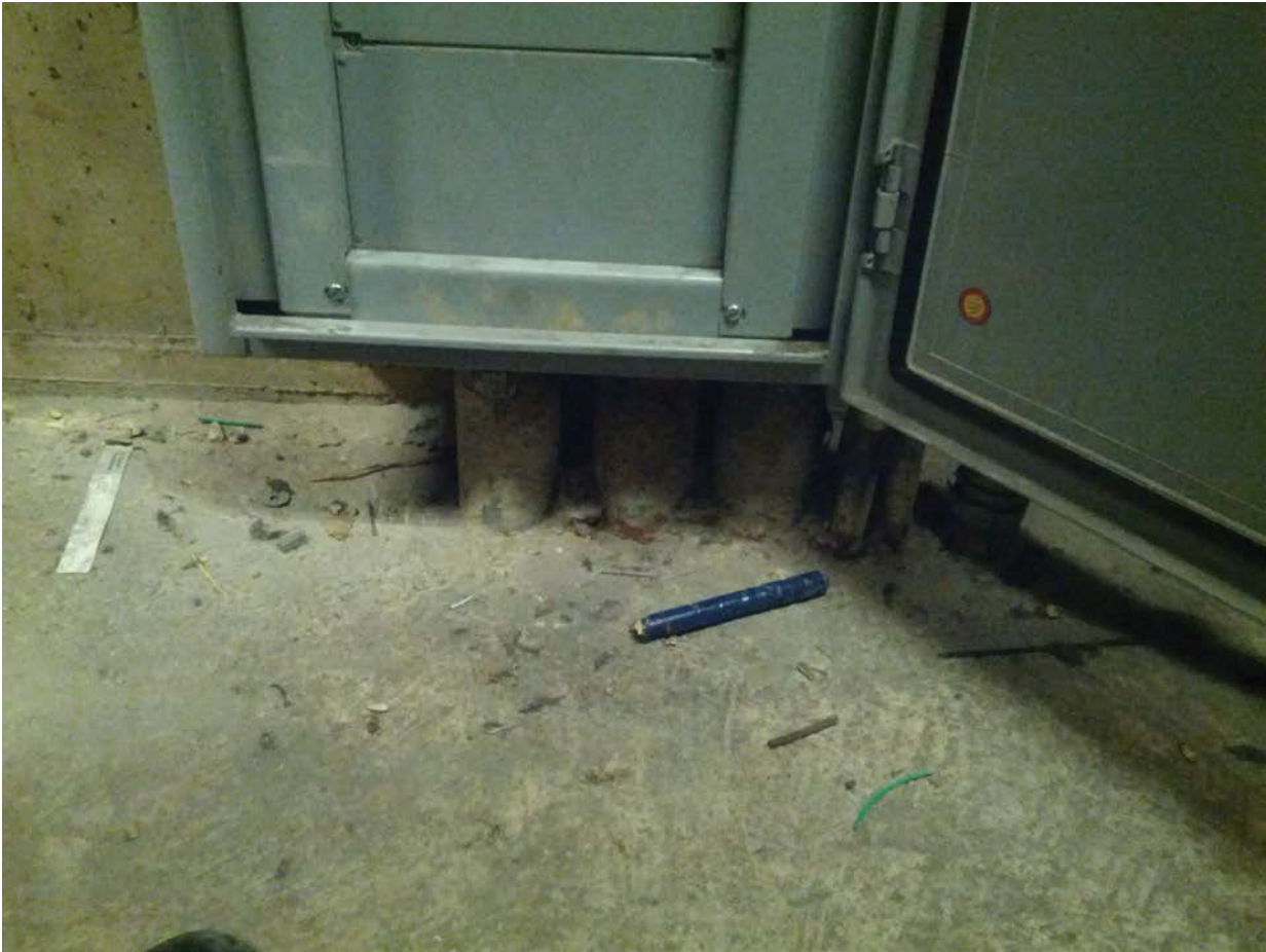
Picture 6: E03 U Street West - AFC Panel WF bottom conduits in Room 212
